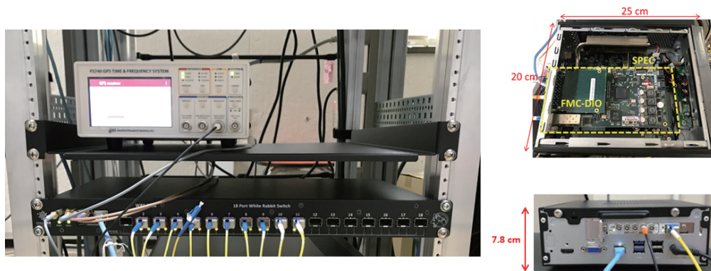
Figure 3.9: White Rabbit modules: the upper white module in the left figure is the GPS receiver. The black 1U-height module under it is the grand-master module of White Rabbit timing system. The right two pictures show the slave node. The PCI Express type slave module is inserted into the commercial PC. The individual slave nodes are connected with the grand-master module via the single mode optical cable.
