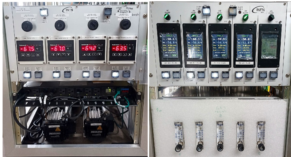
Figure 3.14: Humidity monitoring system installed in E-hut.
